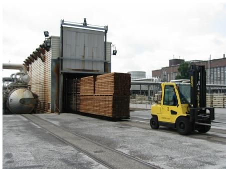
Fig. 3 Industrial kiln for the curing stage
