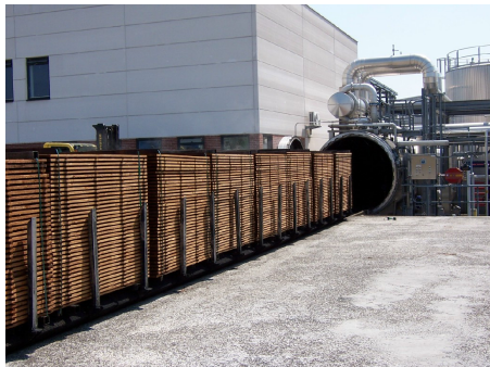
Fig. 1 Industrial plant for the hydro-thermolysis stage
